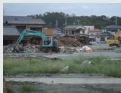
Six months on from the earthquake, excavators were still working every day to clear the damaged homes.
